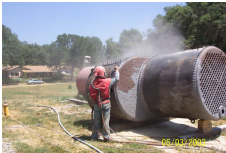
Under the sandblasting helmet is another volunteer, Alan Hiatt. 2,800 lbs of sand and 11 hours later and a boiler appears.
