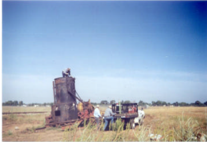
John on top of boiler removing skirting with the careful supervision of Bill and Jim
